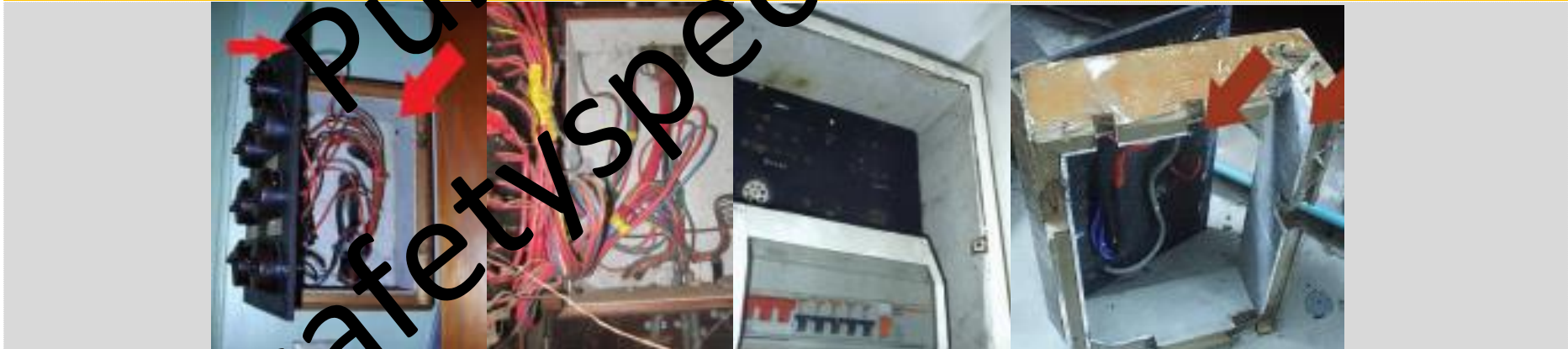
Figure 2: Asbestos cement and asbestos insulation mixed linings inside the electrical box itself.
