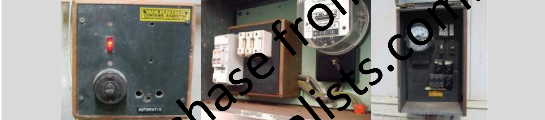
Figure 1: Asbestos based resin mounting boards used across Australia.
